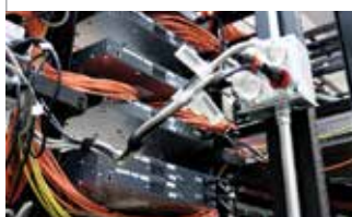
Cable run in server room.
